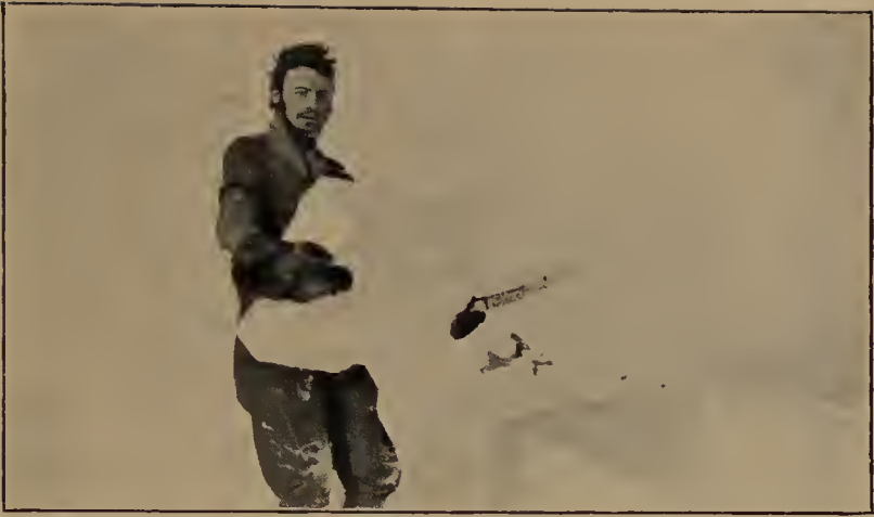
CRAWFORD WITH A BLOCK OF SNOW HE HAS JUST CUT FOR THE HOUSE BEING BUILT BY KNIGHT.
